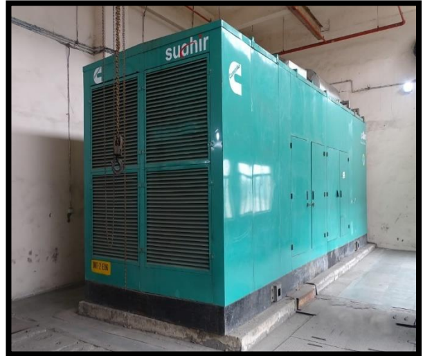
Pic-2 Acoustic enclosure provided at Diesel Generator.
