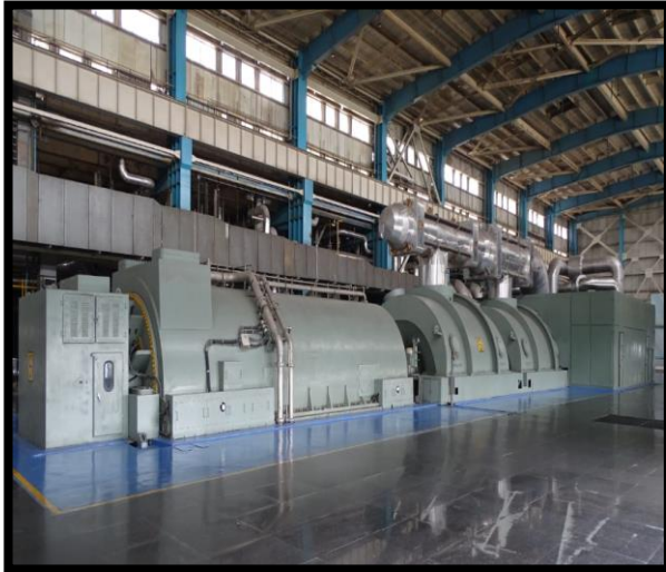
Pic-1 Acoustic enclosure provided at Turbine Generator.
