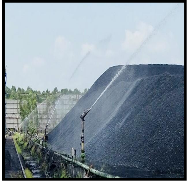
Pic-2 Dust suppression (sprinkler system) provided at each coal stockpile to arrest Dust.
