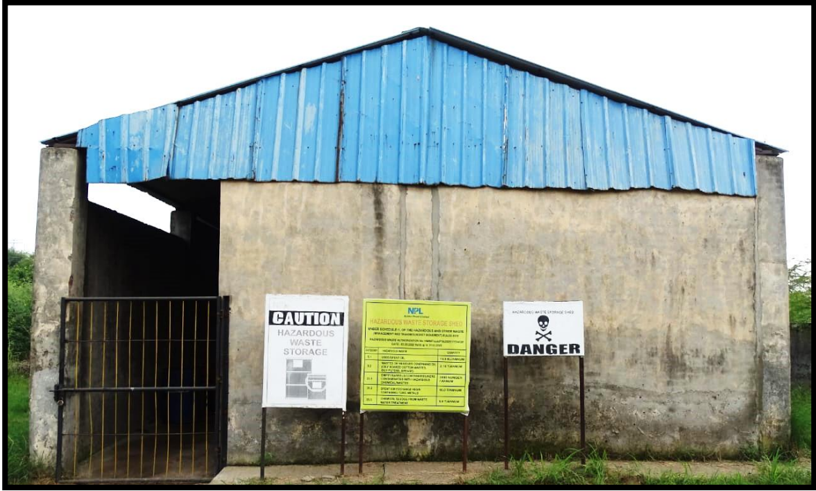
Pic-1 Hazardous waste storage shed to collect and store Hazardous waste generated from plant.
