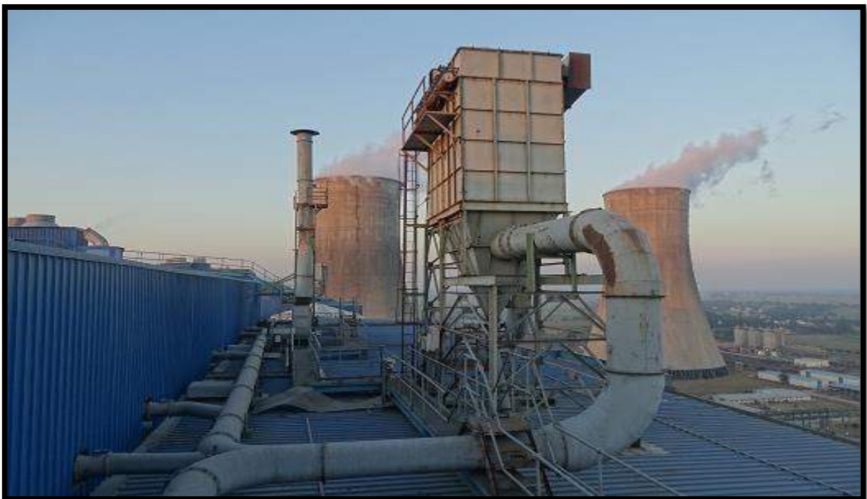
Dust Extraction System at Bunker
