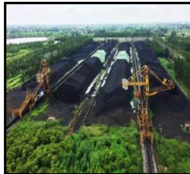
Three side covered windscreens to control fugitive emissions due to wind flow
