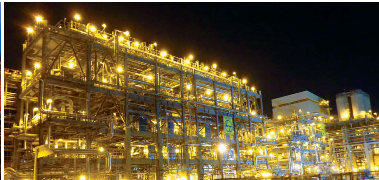
Solution Polyethylene and Specialty Elastomers package for Sadara Chemical Company (JV of Saudi Aramco and Dow Chemicals) at Al Jubail, Saudi Arabia
