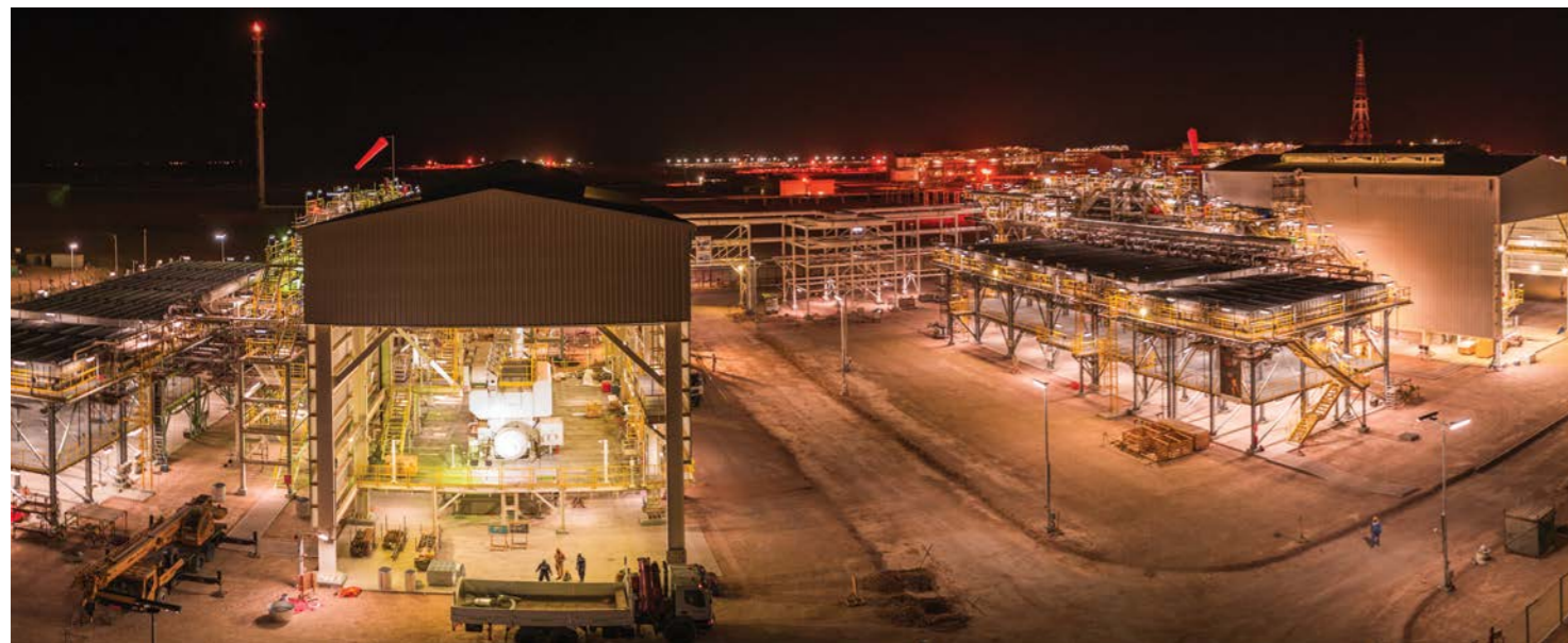
Panoramic view of Saih Nihaydah Gas Compression Project (SNDC2) for Petroleum Development Oman (PDO). The Company has also built PDO's gas processing facilities at Lekhwair, Saih Rawal, Yibal and Kauthar in Oman
