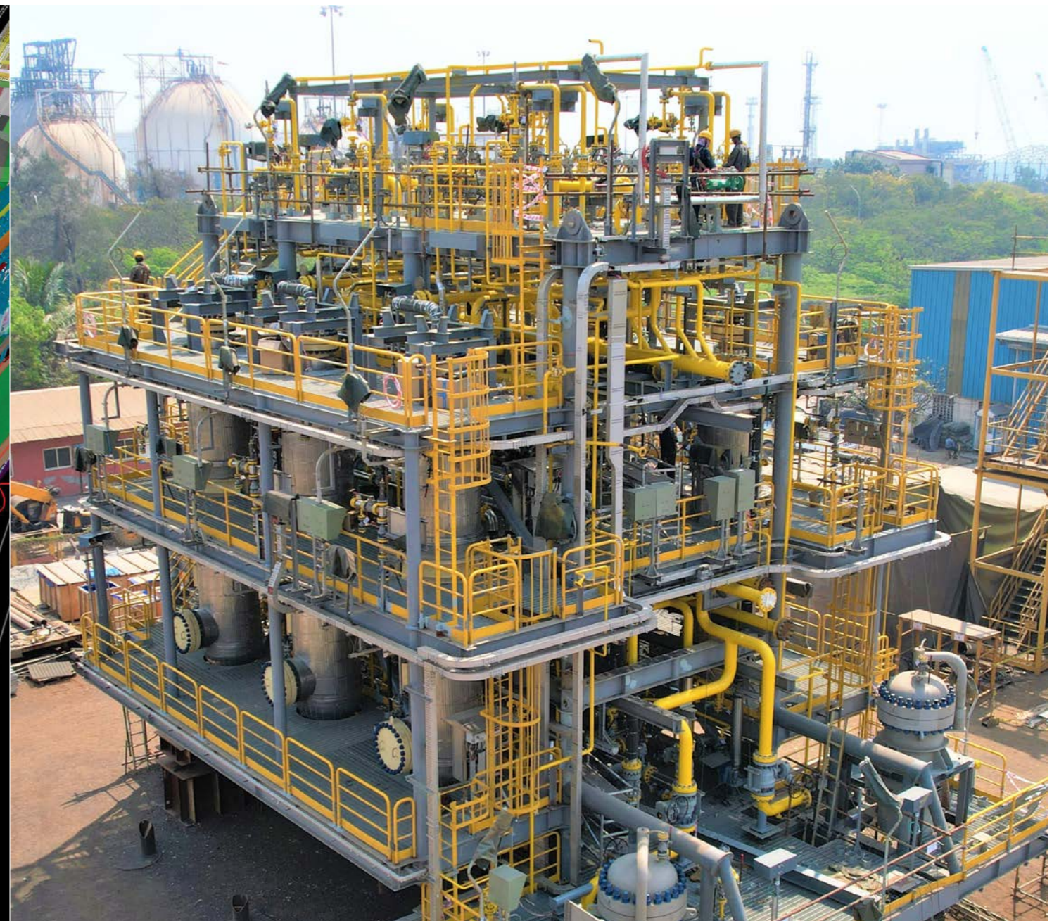
Integrated Module for FPDO Topside - H 2 S Management System
