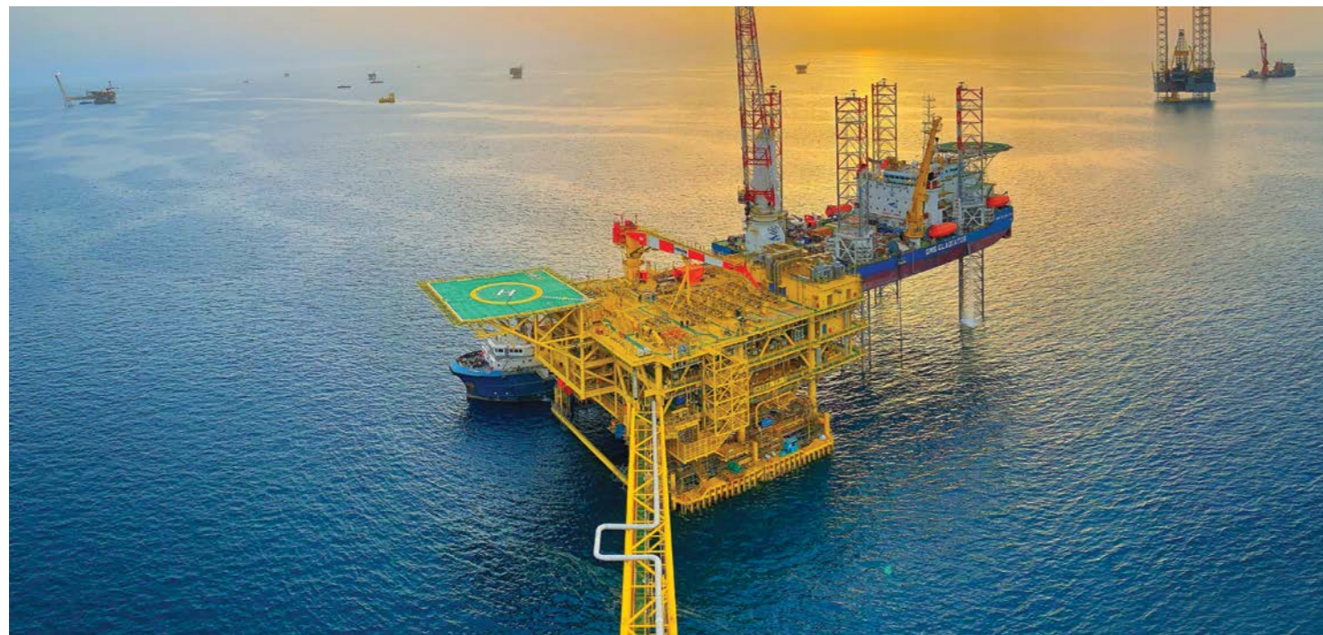
Fully integrated, heaviest gas platform in Saudi Aramco's history, installed by float-over method at Hasbah Field in Saudi Arabia
