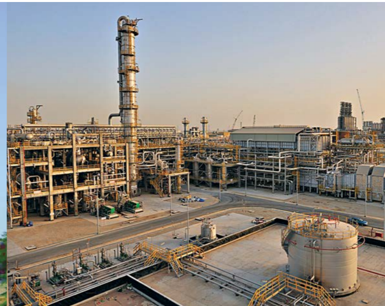
700 TPD Methanol & 100 TPD Carbon Monoxide Plant for Methanol Chemicals Company (Chemanol) at Al Jubail in Saudi Arabia.
