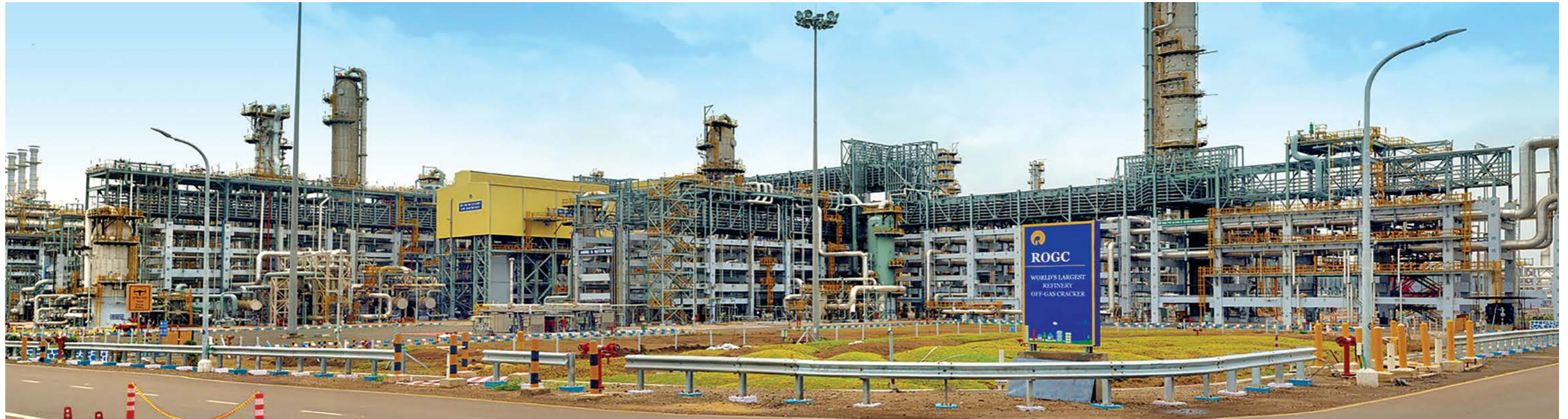
The world's largest ethylene cracker (1.4 MMTPA) – one of multiple systems supplied, installed and pre-commissioned for Reliance's J3 Program, Jamnagar, India. This ethylene cracker is part of the ROGC (Refinery Off Gas Cracker), the heart of C2 Complex
