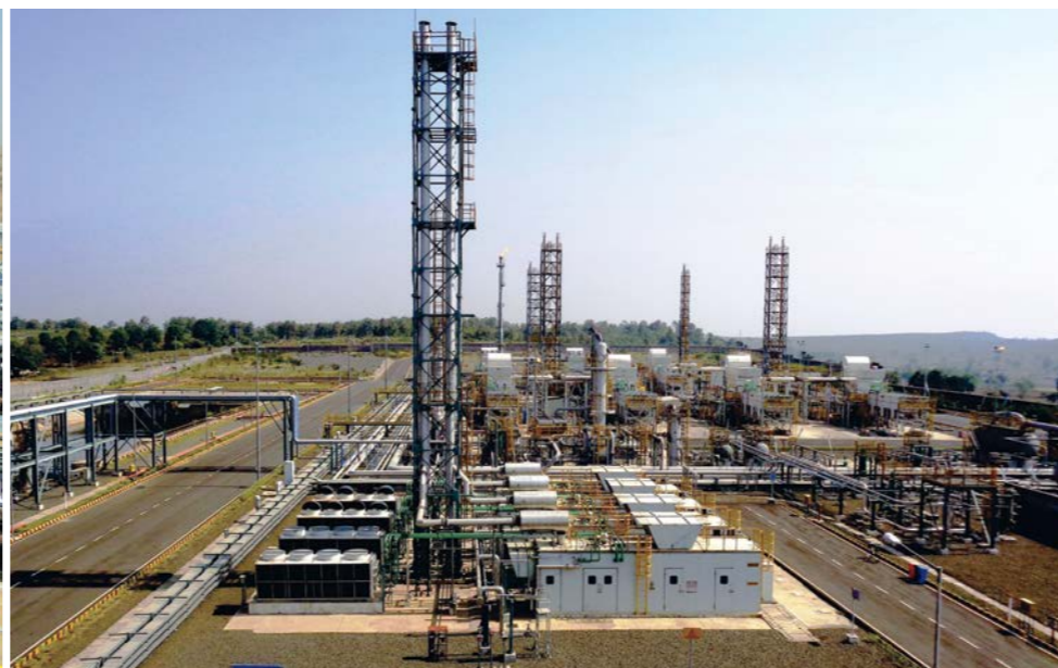
Group Gathering Station-11 for RIL's Coal Bed Methane Field Development Project, Shahdol, Madhya Pradesh
