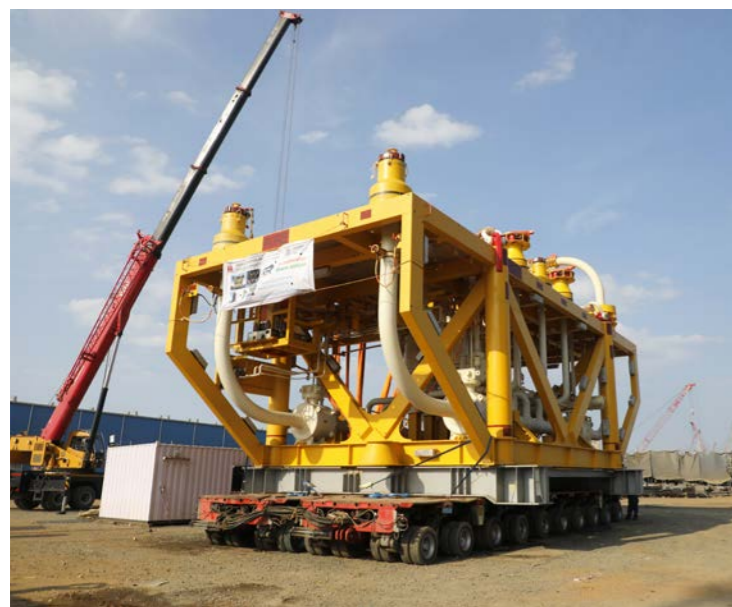
Deepwater Manifold Module for ONGC's KG-DWN-98/2 Project, Offshore India East Coast
