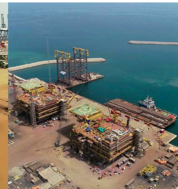
Two mega tie-in platforms (7000 MT each) for Saudi Aramco under fabrication at Oman Facility
