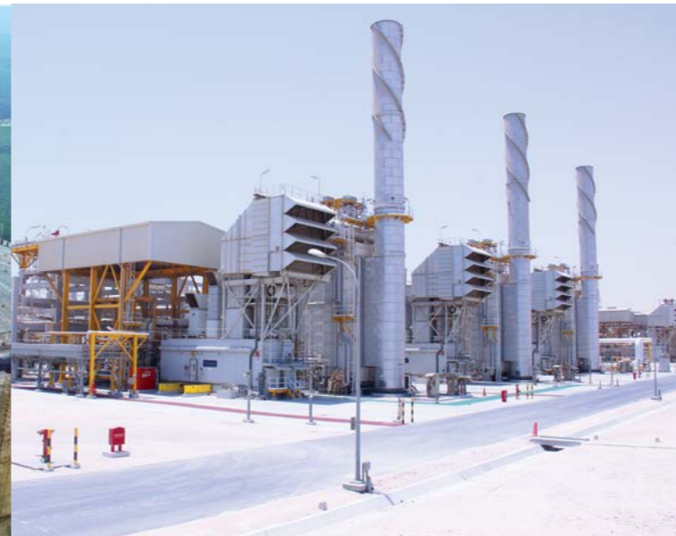
Export Gas Compression Facilities Upgrade Project for Dolphin Energy Limited, Qatar
