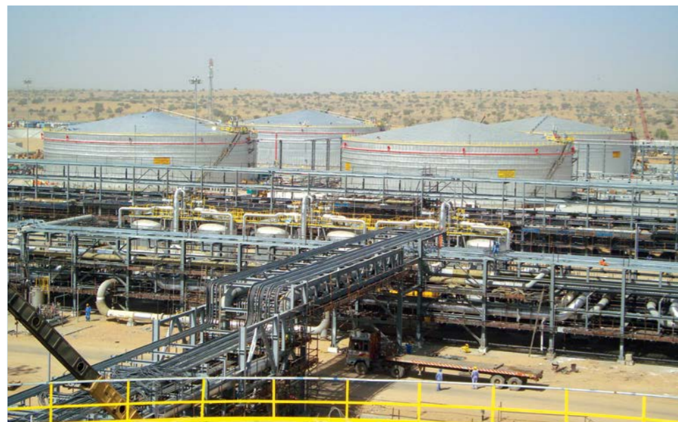
Mangala Process Terminal for Cairn Energy India Limited at Barmer in Rajasthan, India
