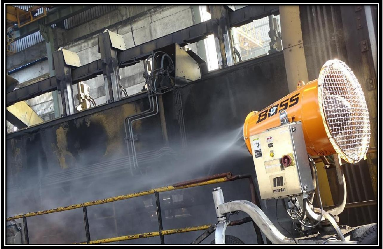
Dust Suppression System installed at Wagon Tippler Area to control Fugitive Emission During Unloading of Coal.
