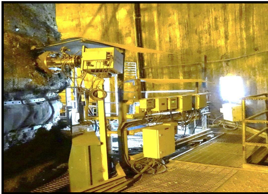
Continuous emission monitoring system installed at main stack for measurement of Particulate Matter & Gaseous Emissions.
