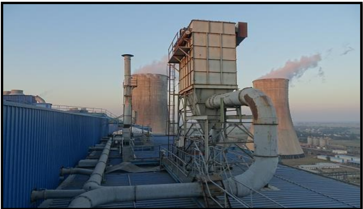
Dust Extraction System at Bunker
