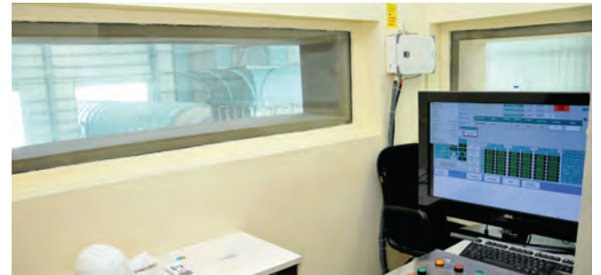
Fan testing control room at L&T Howden's Hazira facility
