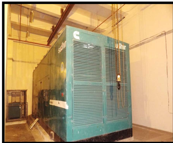
Pic-2 Acoustic canopy provided at Diesel Generator.
