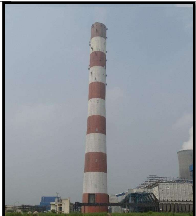
Pic-2. 275-meter-high Boiler stack for wider dispersion of dust and gaseous emissions
