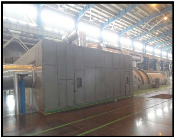
Pic-1 Acoustic Enclosure provided at Turbine Generator.
