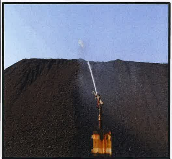
Pic-2 Dust suppression (sprinkler system) provided at each coal stock pile to arrest Dust
