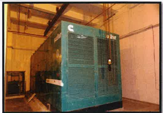
Pic-2 Acoustic canopy provided at Diesel Generator
