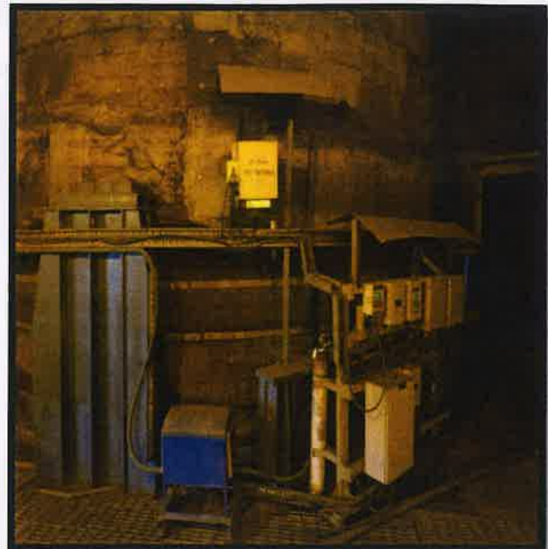
Pic-2 Continuous Emission Monitoring System (CEMS) installed at main stack for measurement of Particulate Matter & Gaseous Emissions.
