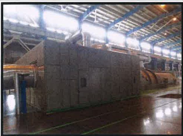
Pic-1 Acoustic Enclosure provided at Turbine generator
