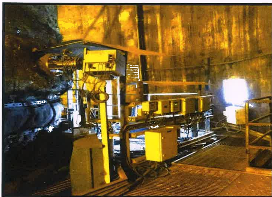
Continuous emission monitoring system installed at main stack for measurement of Particulate Matter & Gaseous Emissions.
