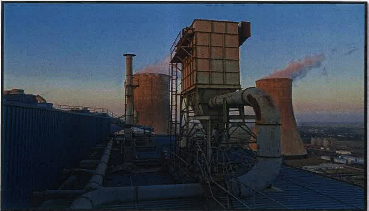
Dust Extraction System at Bunker
