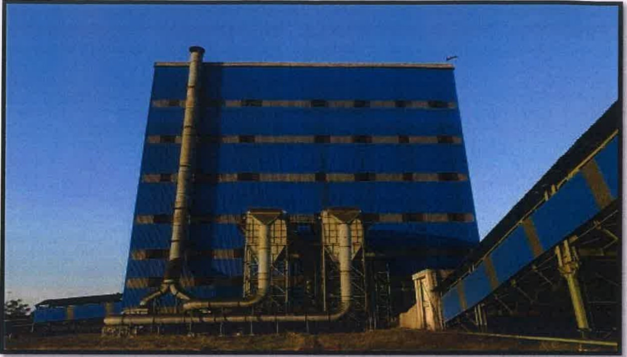
Dust Extraction System at Crusher House
