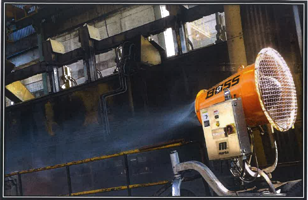
Dust Suppression System installed at Wagon Tippler Area to control Fugitive Emission During Unloading of Coal.
