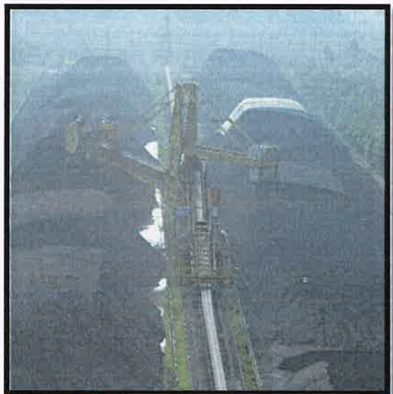
Three side covered windscreen to control fugitive emissions due to wind flow
