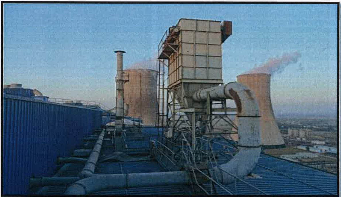
Dust Extraction System at Bunker
