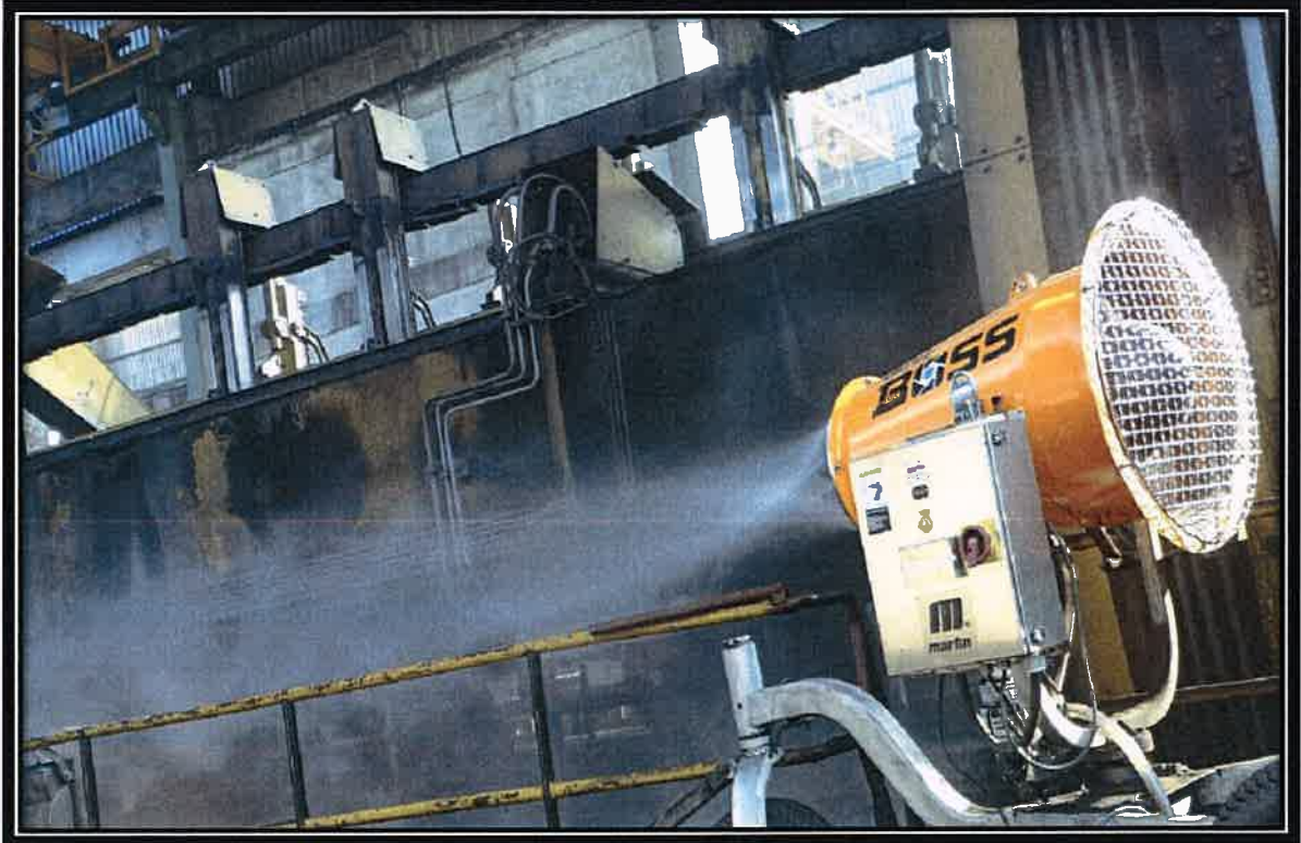
New Dust Canal System installed at Wagon Tippler Area to control Fugitive Emission During Unloading of Coal.
