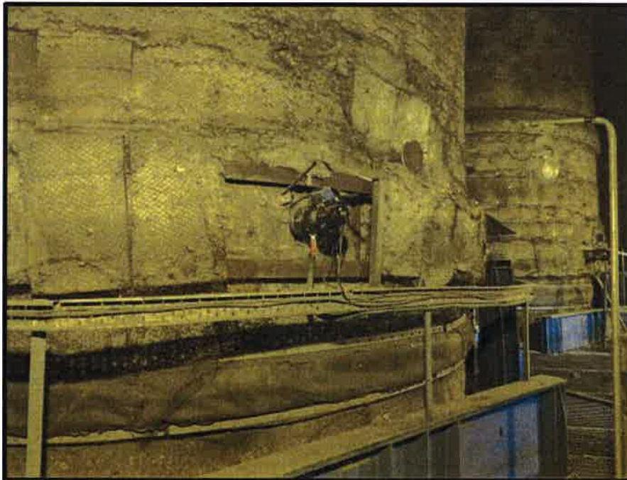
Continuous emission monitoring system installed at main stack for measurement of Particulate Matter & Gaseous Emissions.
