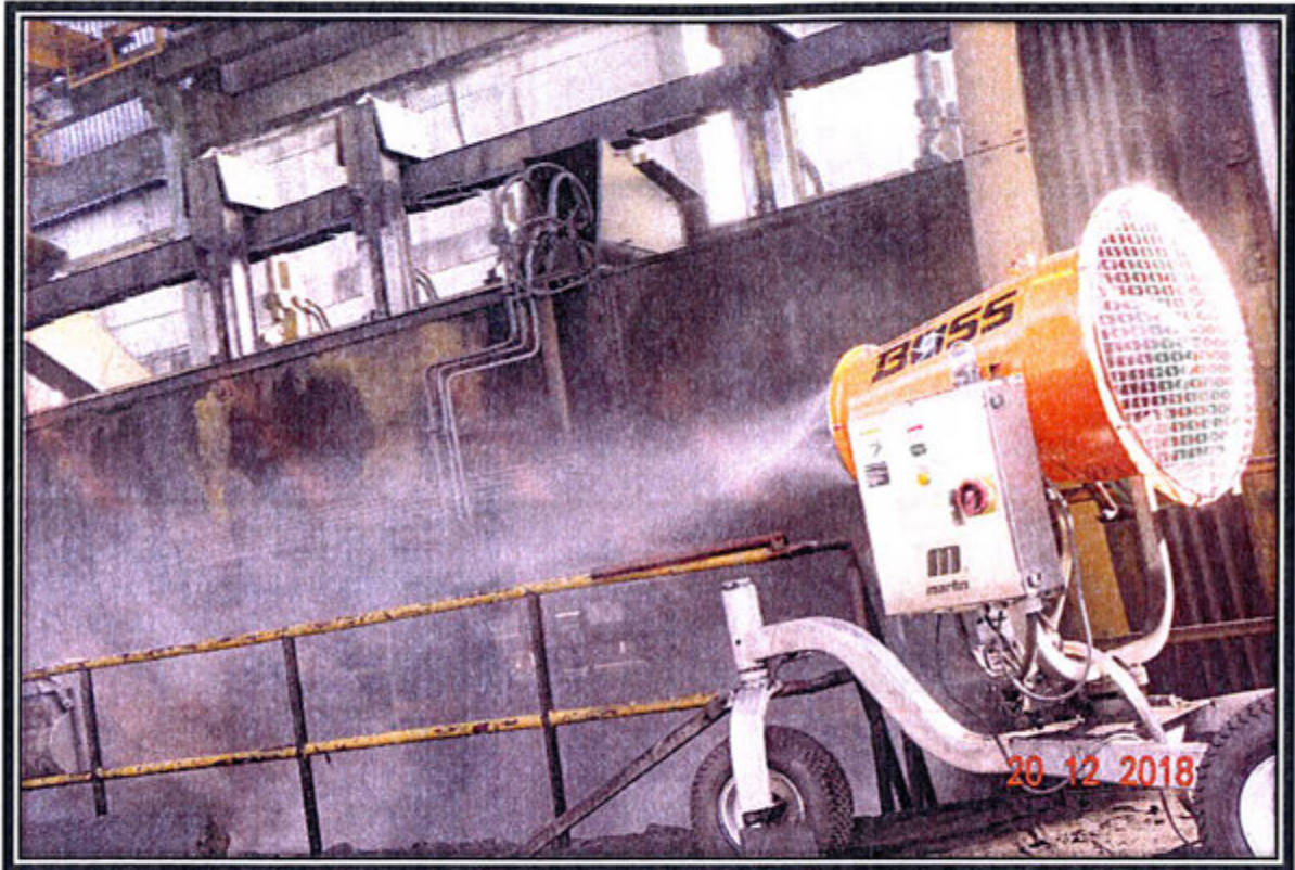
New Dust Canal System installed at Wagon Tippler Area to control Fugitive Emission During Unloading of Coal.
