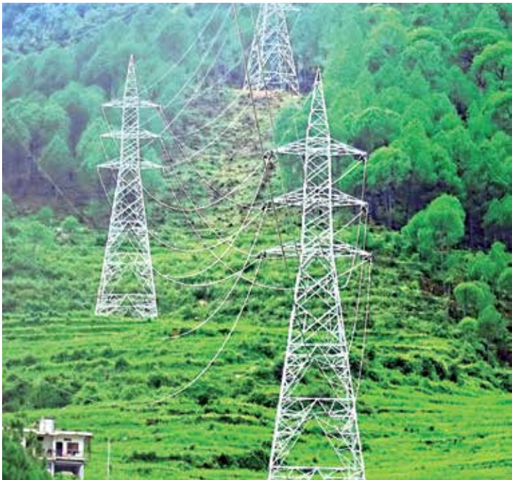
220 kV Uttarakhand Transmission Line
