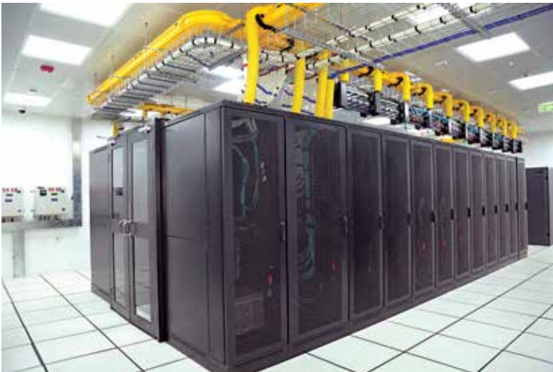
Data Centre for Hyderabad Safe & Smart City
