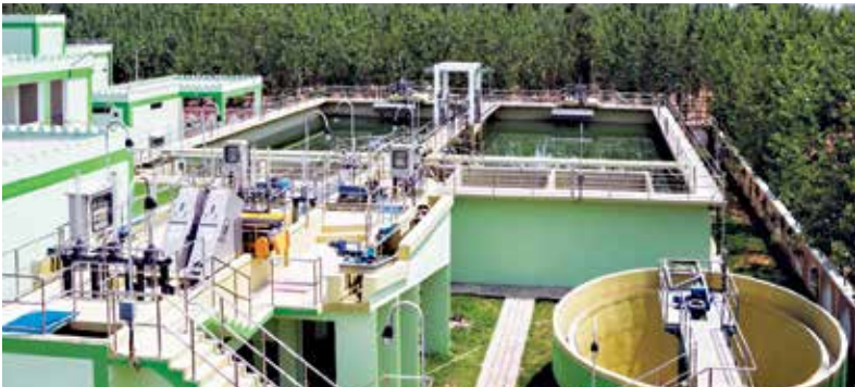
5 MLD Sewage Treatment Plant, Rampur, Uttar Pradesh
