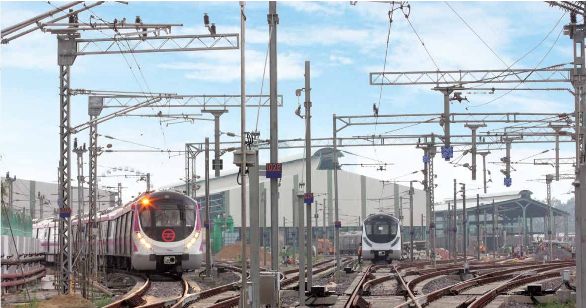
Overhead Electrification for Delhi Metro
