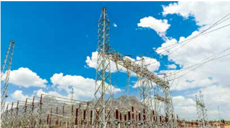
400/132 kV Substation, Nkhoma, Malawi
