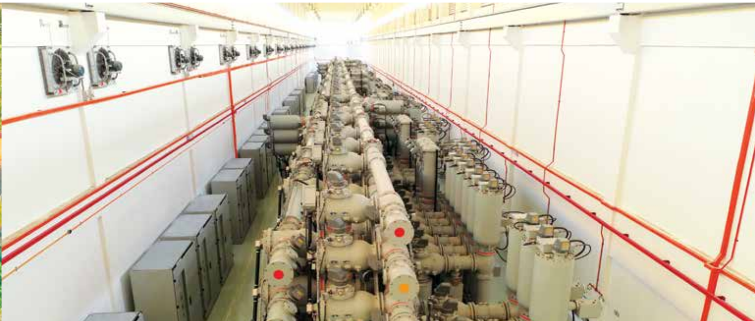
Lambir 275/132-33 kV Gas-insulated Substation, Sarawak, Malaysia
