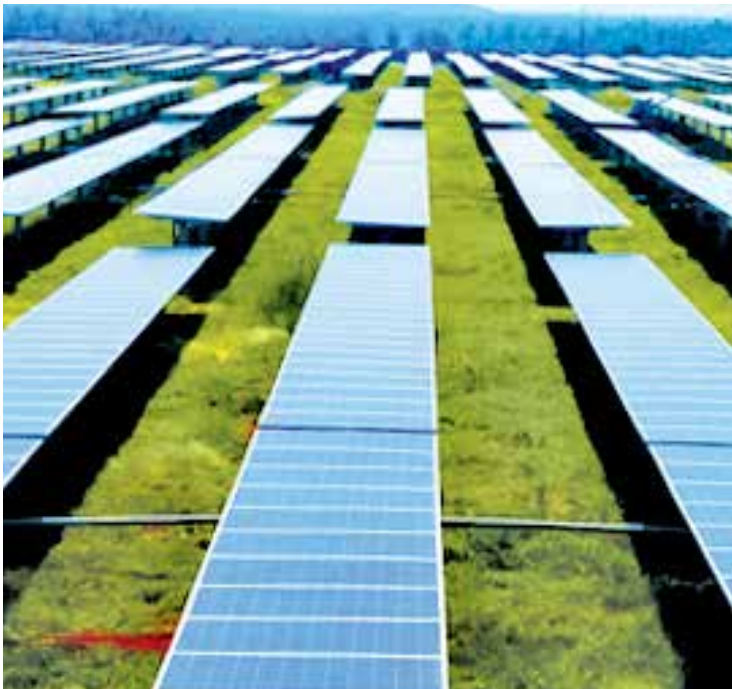
22 MWp HFE Solar PV, Karnataka
