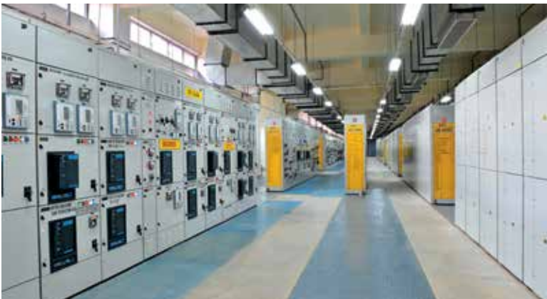
Control Panels at MRPL
