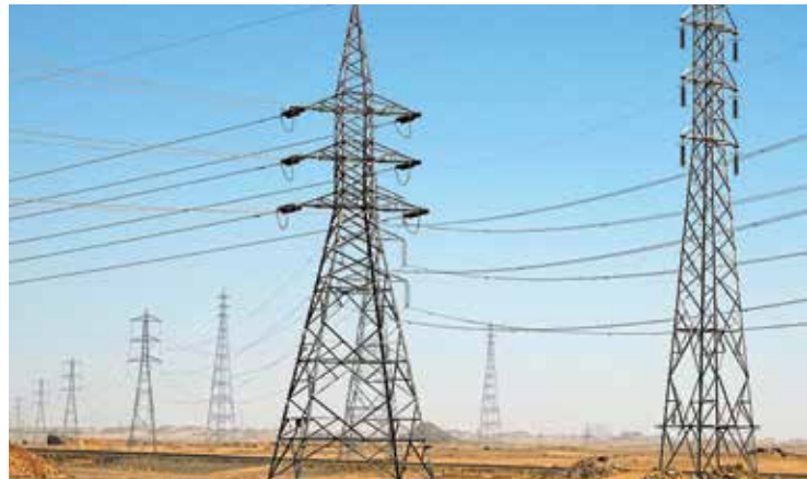
Toshka 2 – Wadi Halfa 220 kV Transmission Line, Egypt
