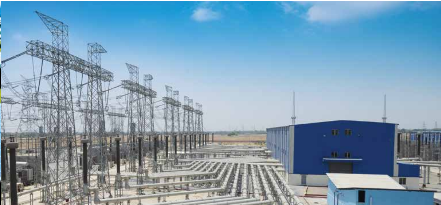
765 kV Gas-insulated Substation, Varanasi, Uttar Pradesh
