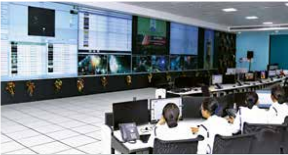
Command & Control Centre, Raipur
