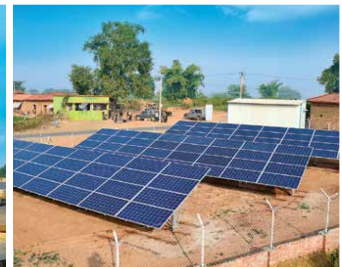
Micro-grid Project for Rural Electrification in Bihar
