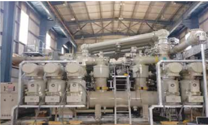
765 kV Gas-insulated Substation, Nizamabad, Telangana
