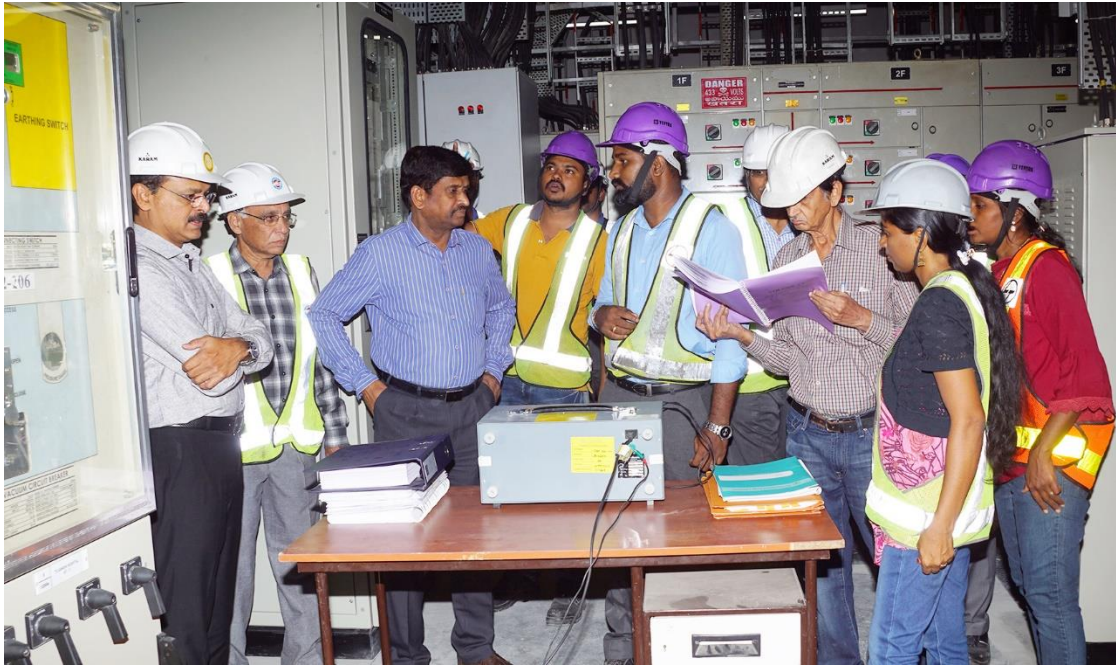
Image 1 - Mr. DVS Raju and Mr. KVB Reddy along with other officials inspecting the Auxiliary Substation Equipment
