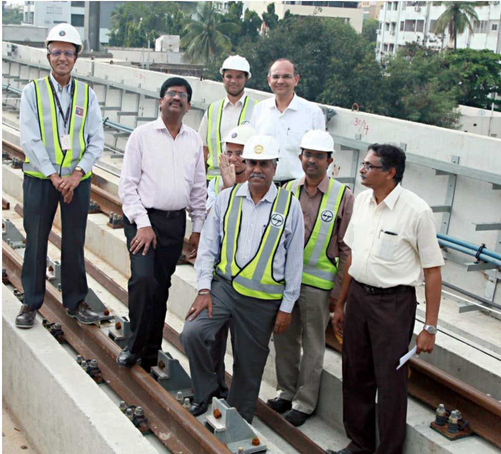
Mr. DVS Raju & Mr. Shivanand Nimbargi (third from left) inspecting the OETS on the viaduct near Begumpet with other team members
