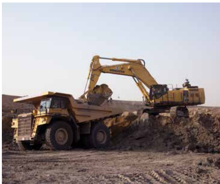
Komatsu PC1250 Hydraulic Excavator loading Komatsu HD785 Dump Truck in opencast project
