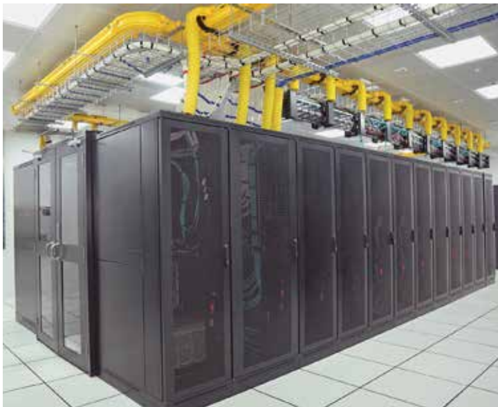
Data Center, Hyderabad
