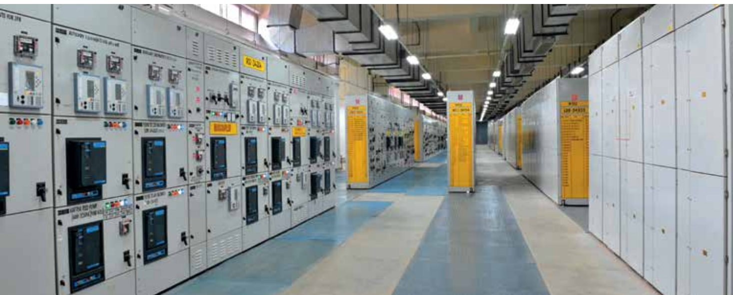
Control panels at MRPL
