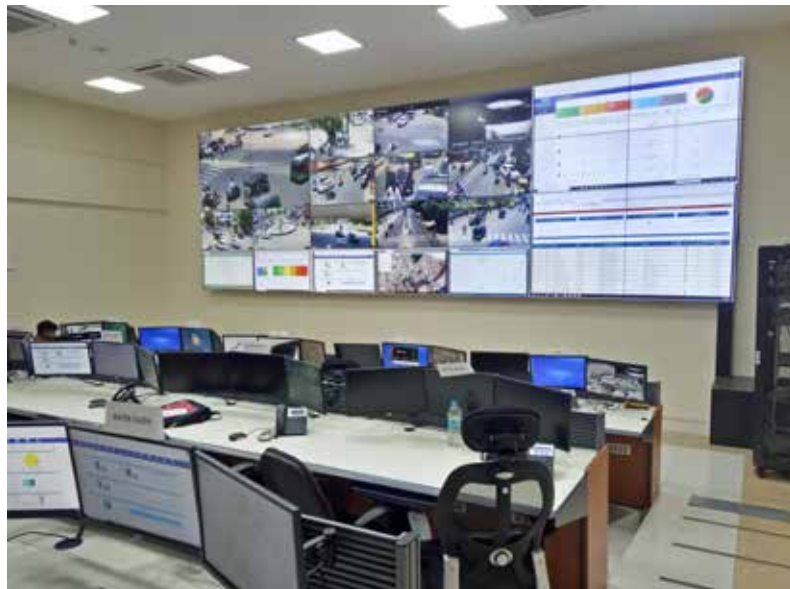
City Command & Control Centre, Vadodara Municipal Corporation
