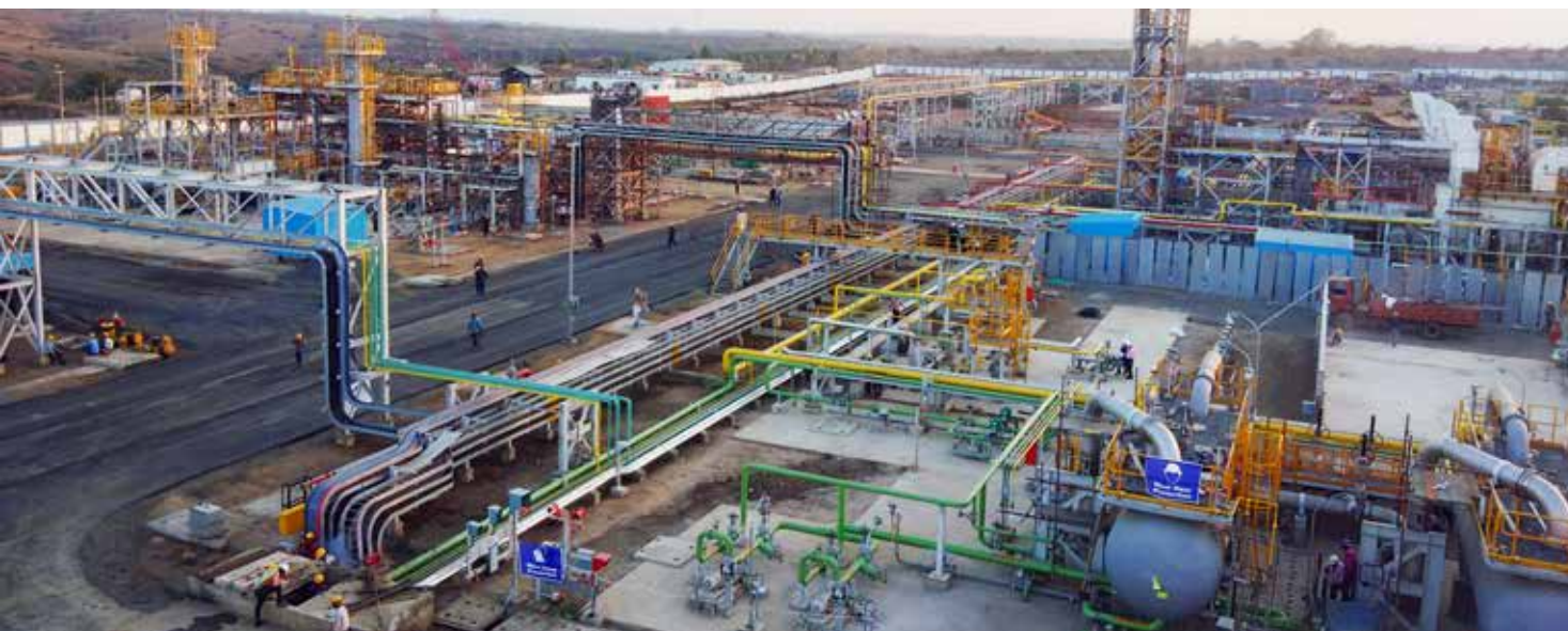
Coal Bed Methane Project (Phase II) for Reliance Industries at Shahdol, India
