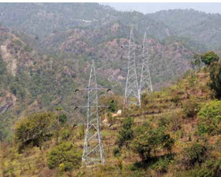
220 kV Transmission Line, Uttarakhand
