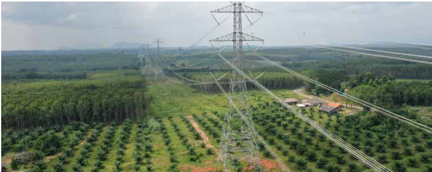
500 kV Bang Saphan-2 to Surat Thani Transmission Line
