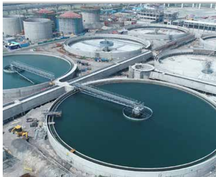
Secondary clarifiers under construction for 318 MLD Waste Water Treatment Plant, Coronation Pillar, New Delhi
