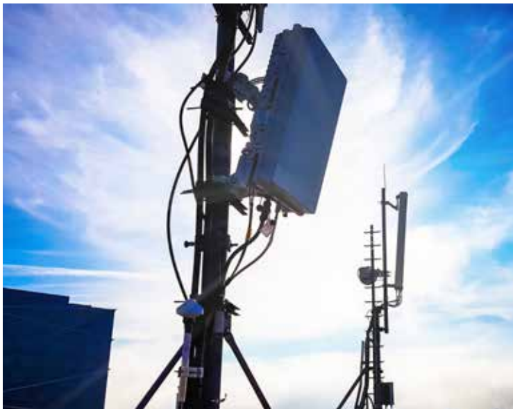
5G Test Solutions are vital in the deployment and success of evolving 5G networks
