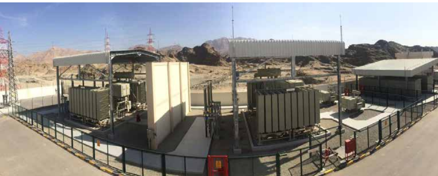
132/133 kV Grid Station at Ghala Heights, Oman
