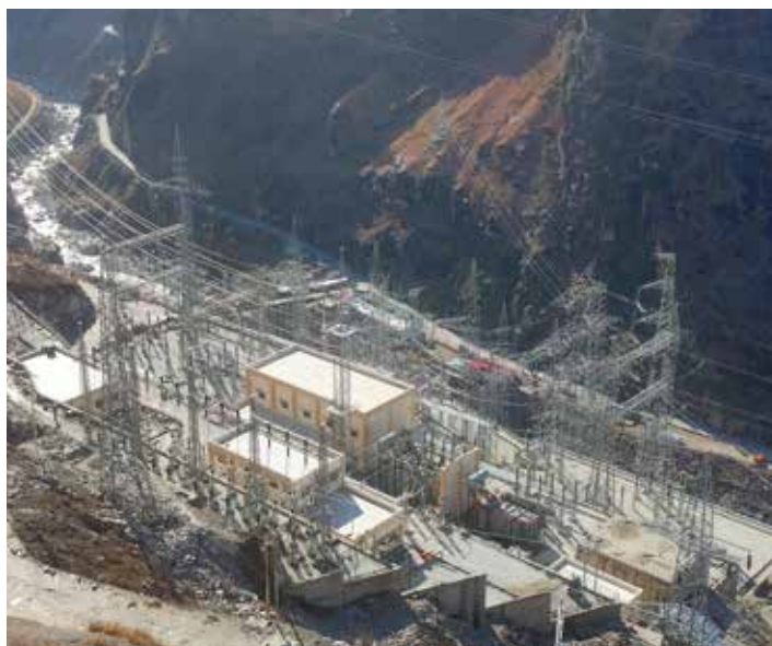
400/220/66 kV Substation at Wangtoo, Himachal Pradesh
