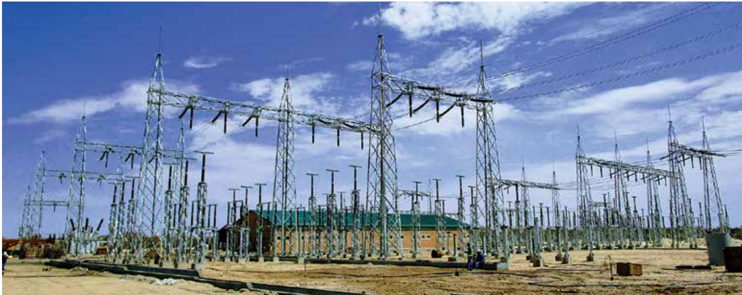
400/220/132/33 kV Substation, Mawana, Botswana
