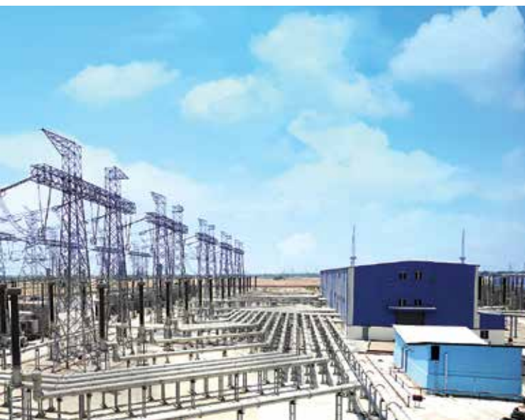
765 kV Gas Insulated Substation, Varanasi, Uttar Pradesh
