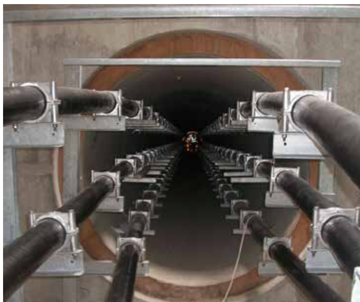
132/33 kV Underground Cable at Ghala Heights, Oman
